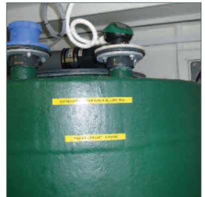
IMP ON CHEMICAL TANK
